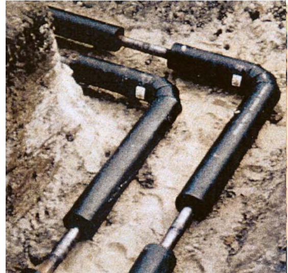
Insapipes Heating Hot Water - direct buried in trench.
