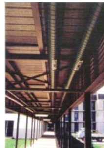
■ Chilled water supported from the casing in covered way
